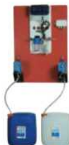
Chemical Dosing for In-Ground Spas
